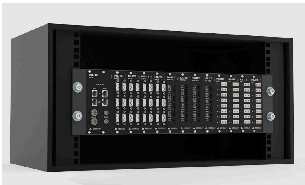
Mounting of IOLITE-R12 in the 19" cabinet
